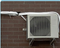
Air Conditioner Condenser Pipe
